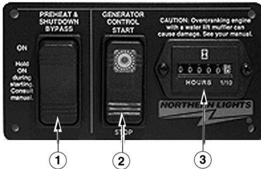
Figure 8: Series 1-B Generator Control Panel
