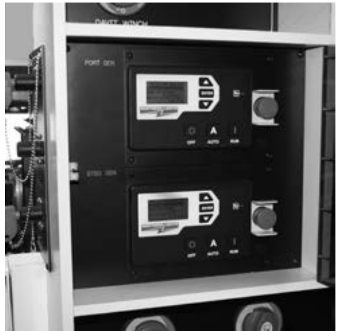
Paralleled TSC panels showing sample installation
